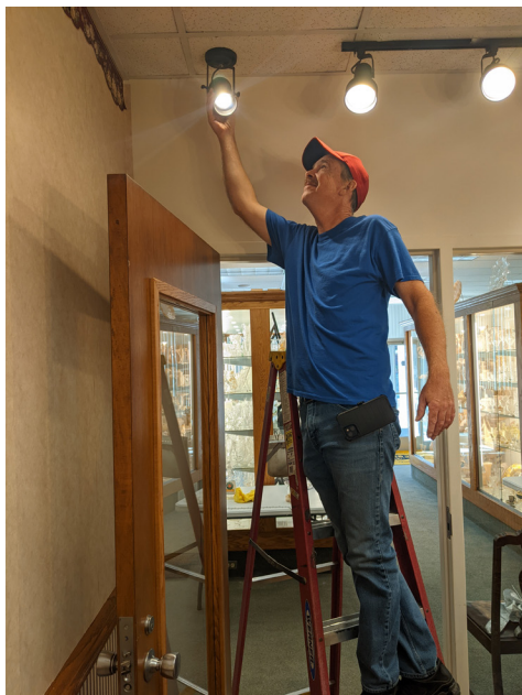
Ben Kirkman, Kirkman's Lighting, installed two additional spotlights in the dining room.
