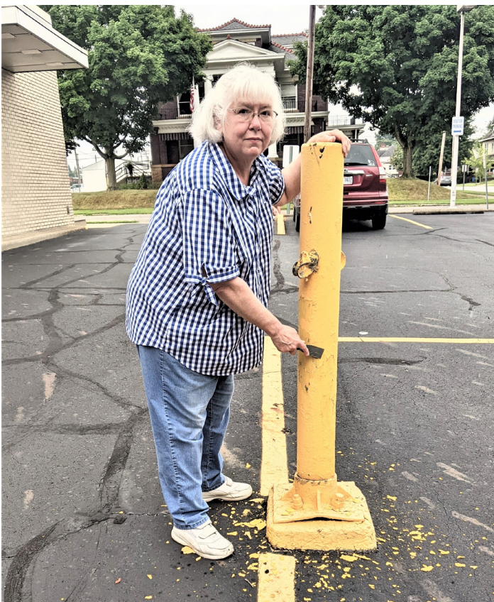
Before the Museum parking lot could be sealed and lined, volunteers scraped the loose paint from the curbs and pole. Lindy Thaxton is shown scraping off layers of paint.
