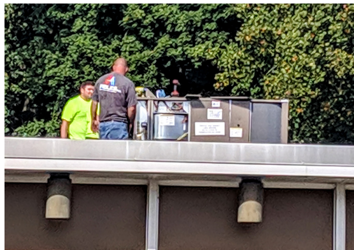
A close up of the Ables team on the roof as the crane moved away from the museum building.
