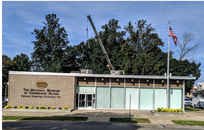
The crane, lifting the new Gas HVAC unit up to the roof, was located behind the museum. Work was done on a Tuesday when the museum was closed.
